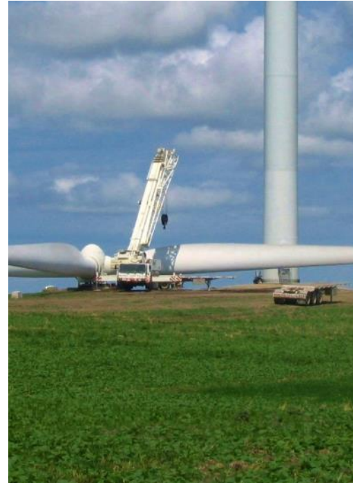
Wind Energy operations
